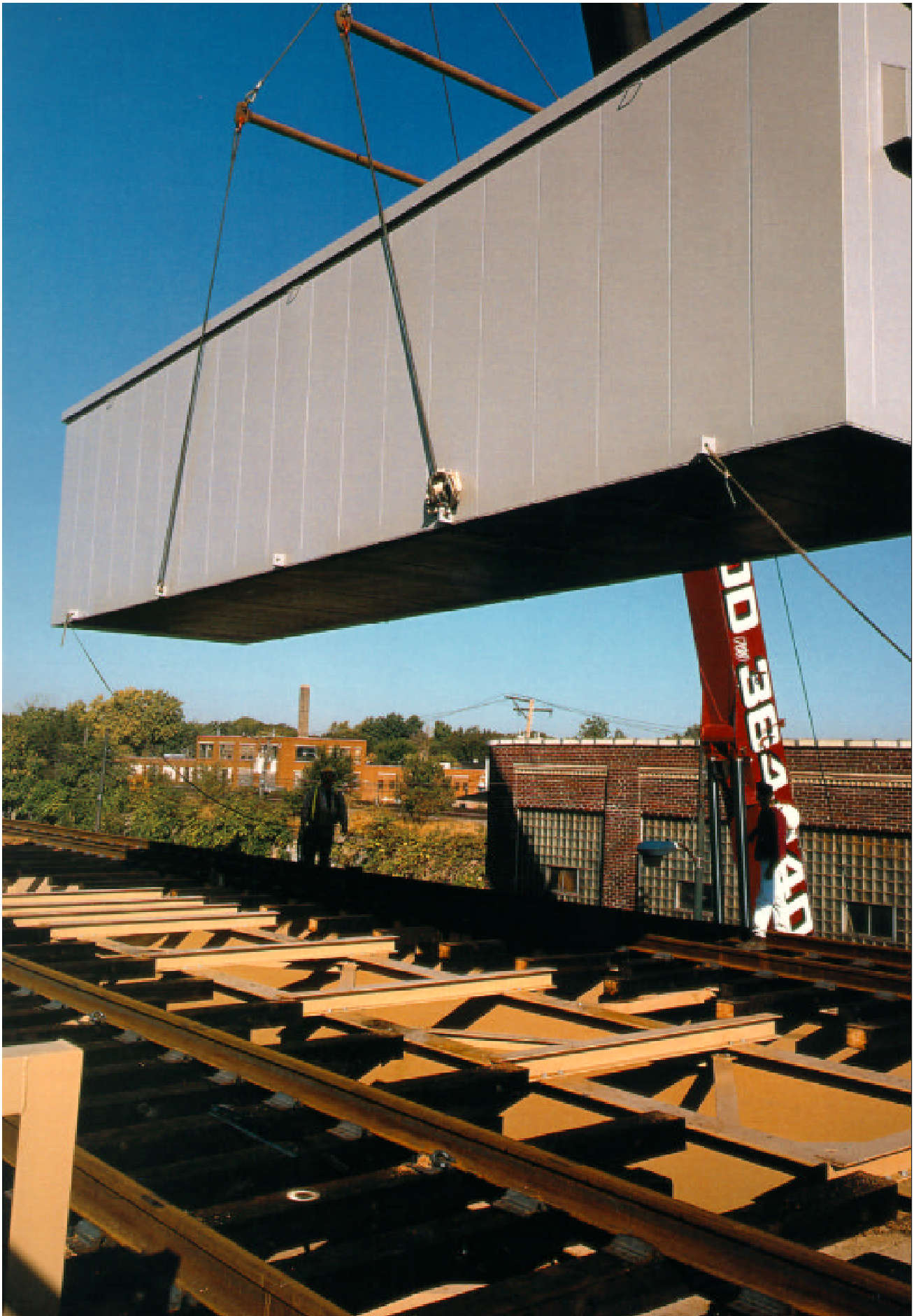
Lowering a bungalow onto the elevated tracks on the "Green Line" rail transit route in Chicago. The bungalow houses the controls that regulate the operation of a portion of the Chicago Transit Authority's renovated system. The $13.5 million "Green Line" project was Harmon's largest rail transit award to date.
